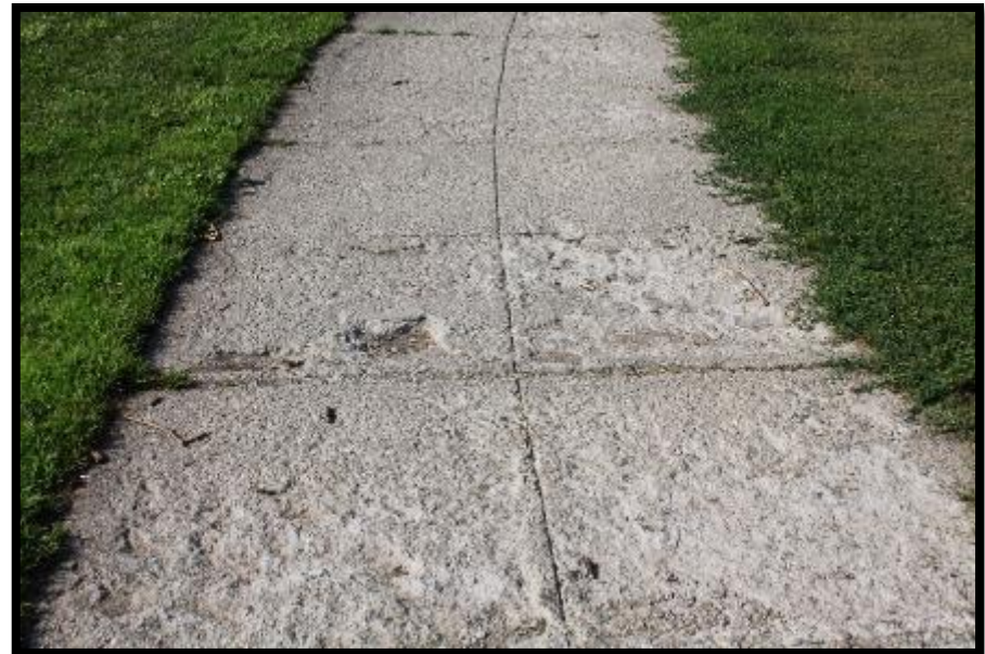
Typical spalling damage
