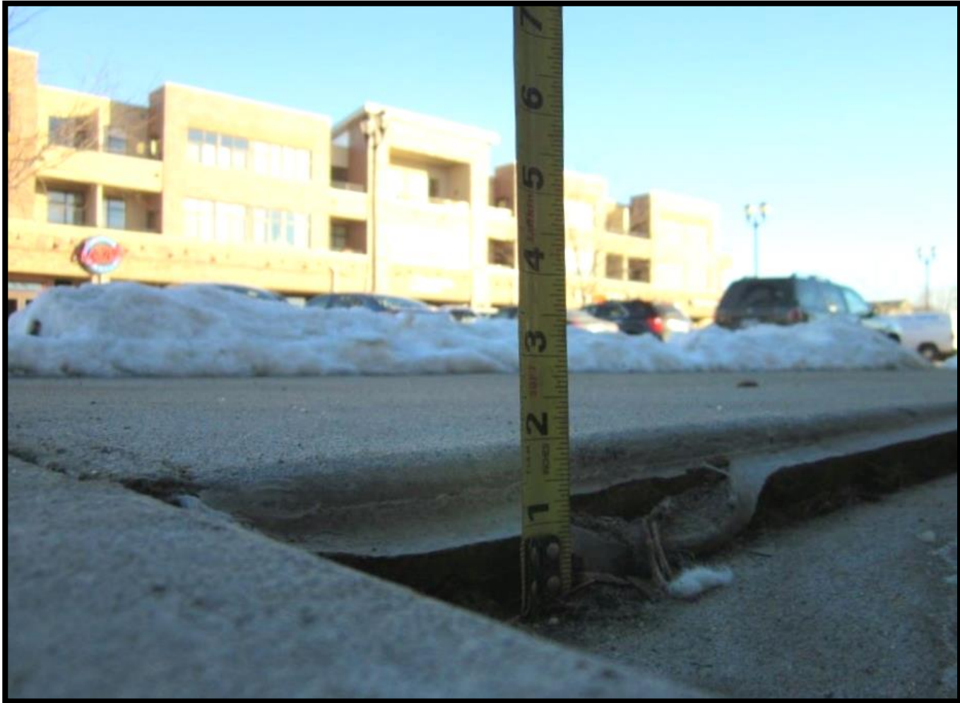
Slab settled 2", broken hand
